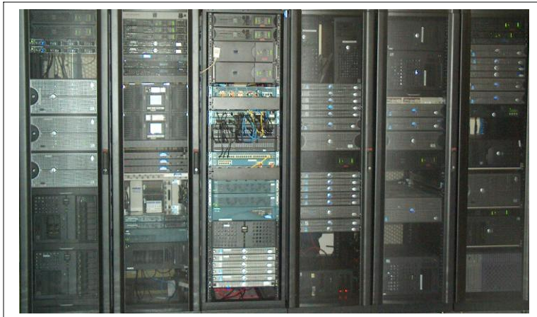
Telephony Servers & Out-Calling Engines
